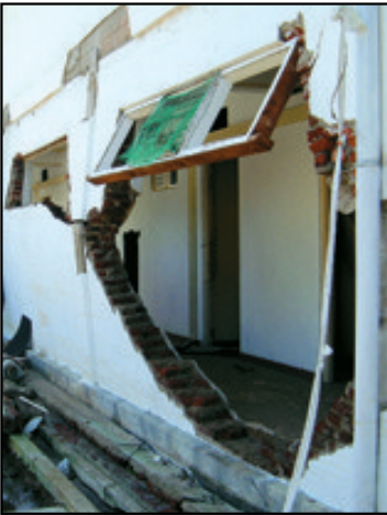
Full force: Destruction of homes and commercial buildings is widespread.
